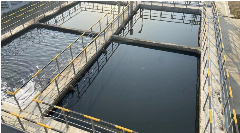
The Sewage Treatment Station at Yibin Brewery
