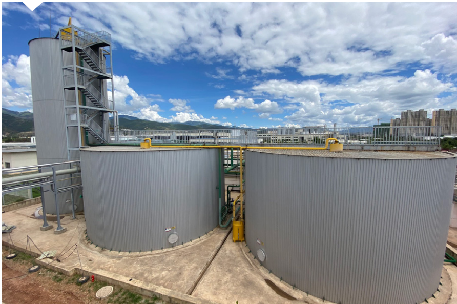
The Reclaimed Water Treatment Plant of Xinjiang Wusu Brewery
